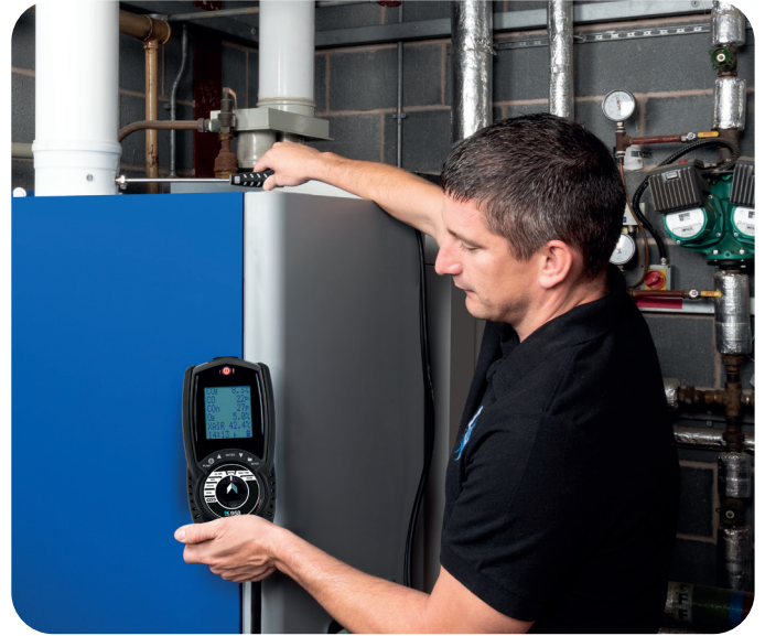
Flue Gas Analysis
